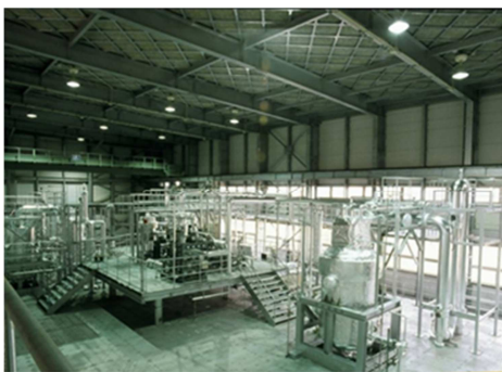
Figure 3: 30 kW OTEC and Desalination Room, Saga-Japan [IOES]
